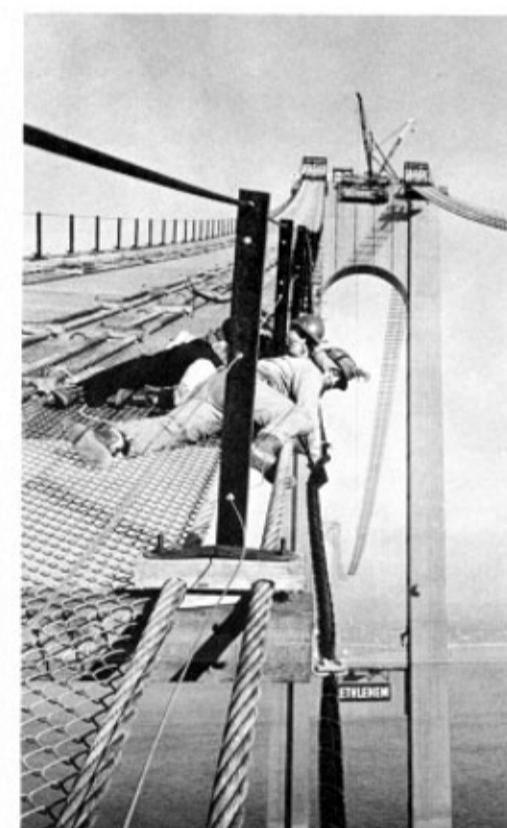
Workers installing the catwalk for the majestic Verrazano-Narrows Bridge preparatory to spinning the cables between Brooklyn and Staten Island anchorages this spring. The $325,000,000 bridge, which will have the largest center suspension span in the world, is a key project in the metropolitan arterial system. By 1965, it will provide a new fast route to the Fair for visitors from south and central New Jersey.
