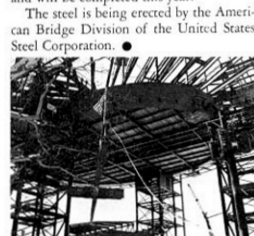
The final section of steel atop the Port of New York-New Jersey Exhibit Building and Heliport at the New York 1964-1965 World's Fair, was lifted into place on January 31. The building will be completed by the end of 1963.
