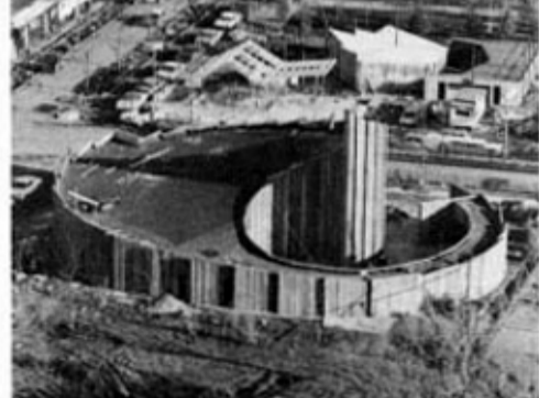
Occupying a site of 6,000 square feet in the International Area, the spiral-shaped American-Israel Pavilion is sheathed in red-wood mahogany. Contractor for the pavilion is Hegeman-Harris Company, New York, N. Y.
