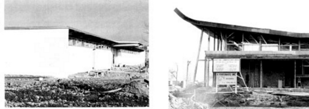
Construction is visibly advancing on the circular structure that will house General Electric's theater and its Walt Disney production. This is among other exciting presentations of MCI's achievements in the field of electricity and electronics. The 56,000 sq. ft. site is in the Industrial Area alongside the Pool of Industry at the intersection of the Avenue of Commerce and Progress.
