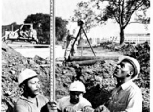
Harris James, Alfonso Maisno and Tom Brown steady a drainage pipe as Joe Lazo at rear checks exact position.
