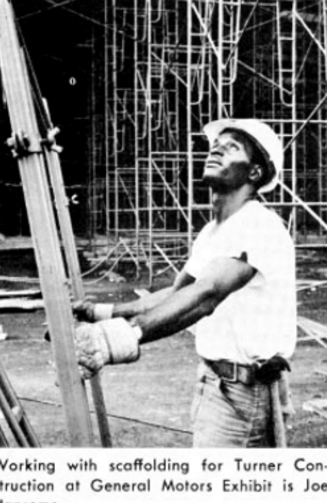
Working with scaffolding for Turner Construction at General Motors Exhibit is Joe Hansome.
