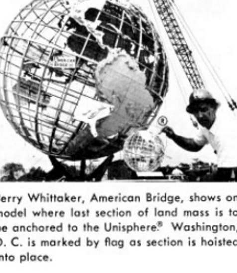
Perry Whittaker, American Bridge, shows on model where last section of land mass is to be anchored to the Unisphere®. Washington, D. C. is marked by flag as section is hoisted into place.
