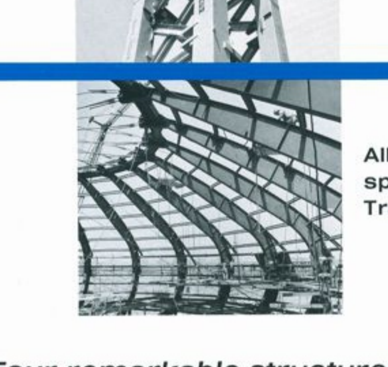
Steel U-frames connected to curving trusses frame the ride for the Bell System Exhibit
