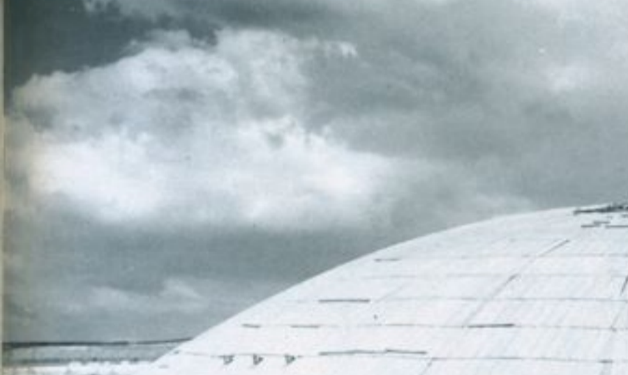
Next step was to erect the upper halves of the ribs (welded splices), and install purlins. Meanwhile, the tension ring was positioned on falsework. When all cables were tensioned, the basic structure was complete.
