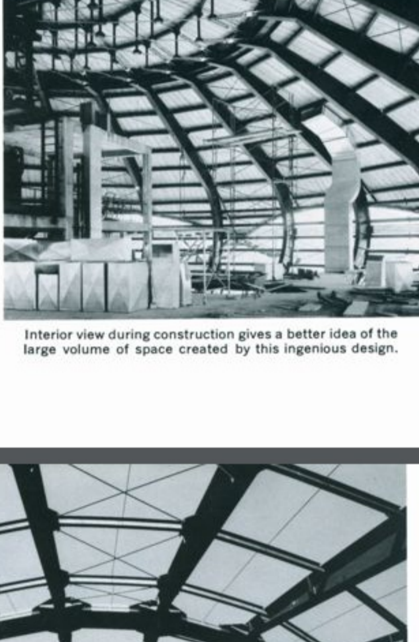
Interior view during construction gives a better idea of the large volume of space created by this ingenious design.
